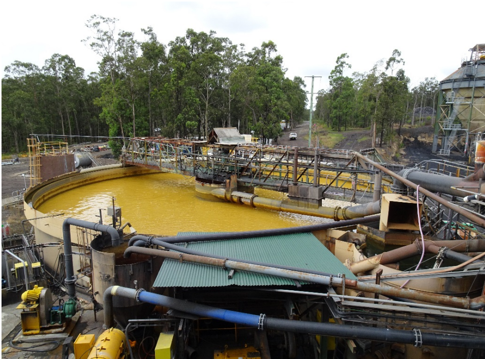
Figure 3: Coal Washing Plant
