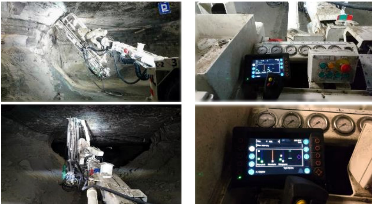
Figure 14:View from bolting mast during bolting process. Optional Bolt Counter System installed. Source: Mine Master
